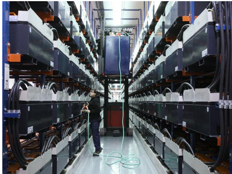
Fairbanks Alaska's backup battery with 13,760 nickel-cadmium cells
